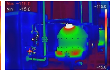
Check Mechanical Status
