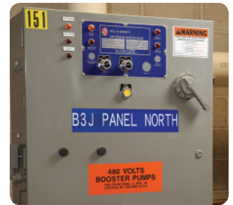
Control Panel & Electrical Panel Labels
