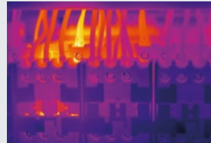
Maintain systems: Identify excessively high temperatures in circuit breakers and electrical components before breakdowns can occur.
