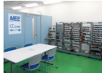
Conformance testing lab
