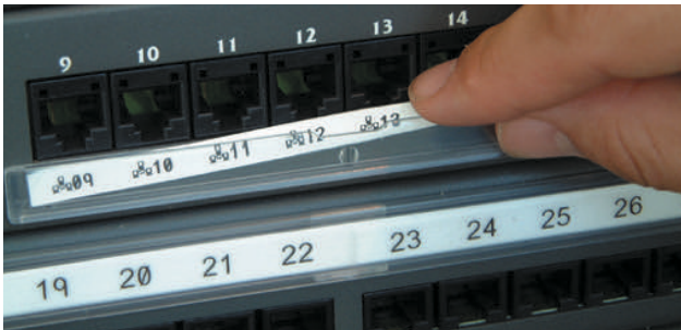
Punch block & patch panel labels
