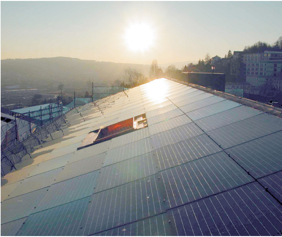
Anlage Application Application Waidspital, Zürich (CH)
