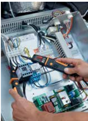
Measuring voltage on a compressor.
