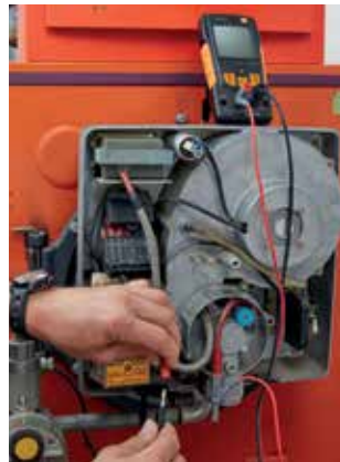
Ionization current measurement set-up
