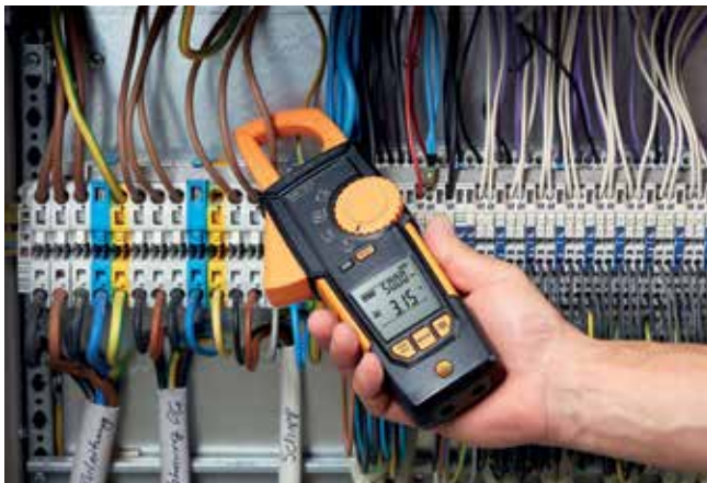
Measuring current in a switching cabinet.
