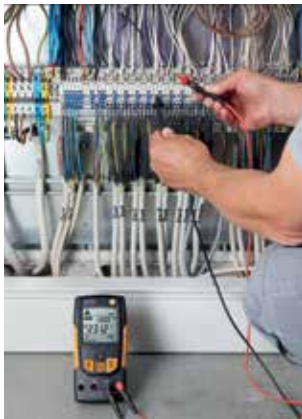
Testing voltage in a switching cabinet.
