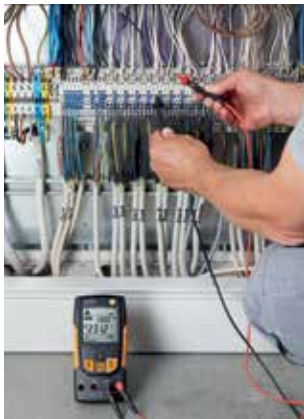
Testing voltage in a switching cabinet.
