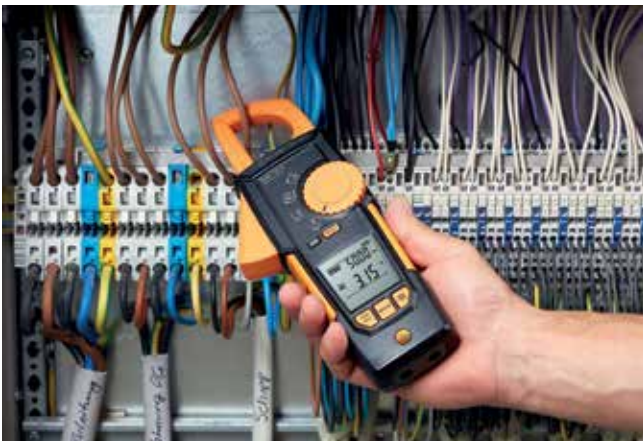
Measuring current in a switching cabinet.
