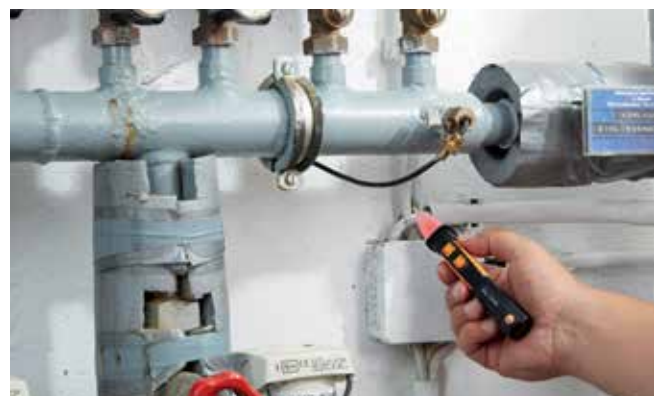
Checking voltage on a distributor box with testo 745 .
