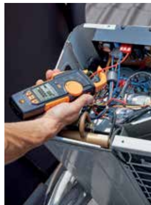
Hooking the clamp meter into an outside refrigeration unit.
