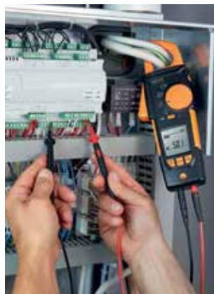
Measuring voltage on the switching box of a heat pump with suspended measuring instrument.
