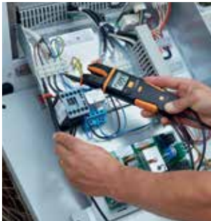
Measuring voltage on a compressor.
