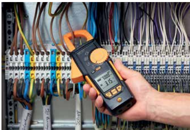
Measuring current in a switching cabinet.
